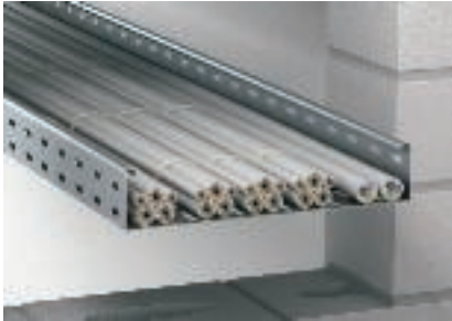
Fixing within a cable tray Bundles of cables in cable trays can be protected against slippage by fixing with cable ties.
